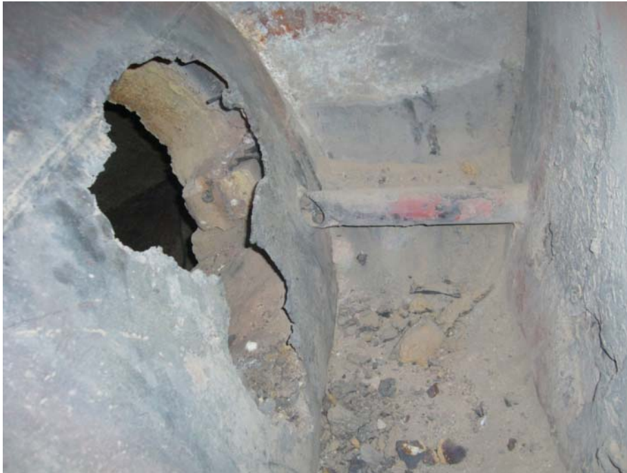
Figure 4-65 – Same as figure above after damage due to oxygen combustion resulting from oxygen injection into the thermal combustor on the front end of the reaction furnace.
