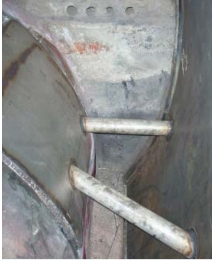
Figure 4-64 – Thermal combustor on the front end of a reaction furnace on a sulfur recovery unit.
