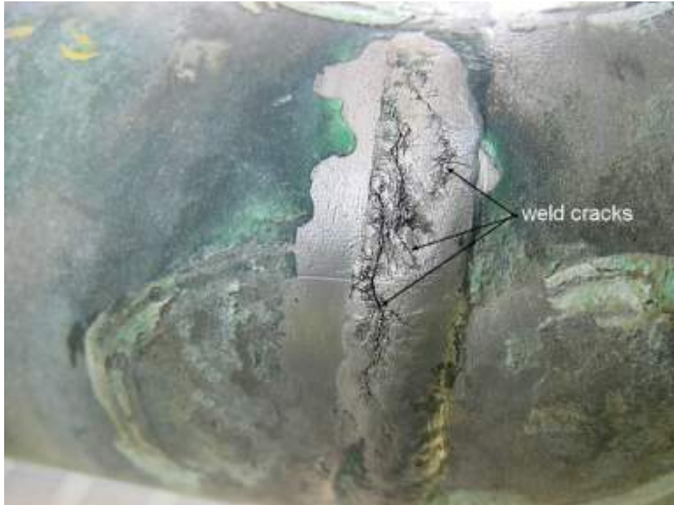
Figure 5-16 – HF stress corrosion cracking of Alloy 400 vent line in an acid dump system (Reference 8).
