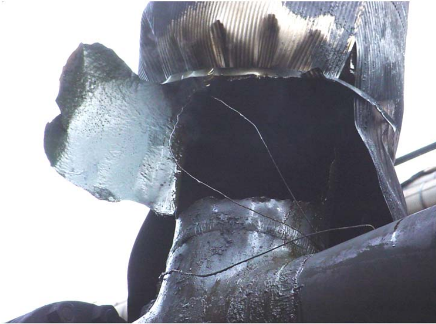
Figure 4-117 – Sulfidation failure illustrating the effect of accelerated corrosion due to low silicon content. This 8 inch NPS pipe section in FCC bottoms piping was in service at 150 psig (1Mpa) at 650° to 700°F (340° to 370°C). The piping sketch in Figure 118 illustrates the difference in corrosion rate as compared to adjacent high-silicon components.
