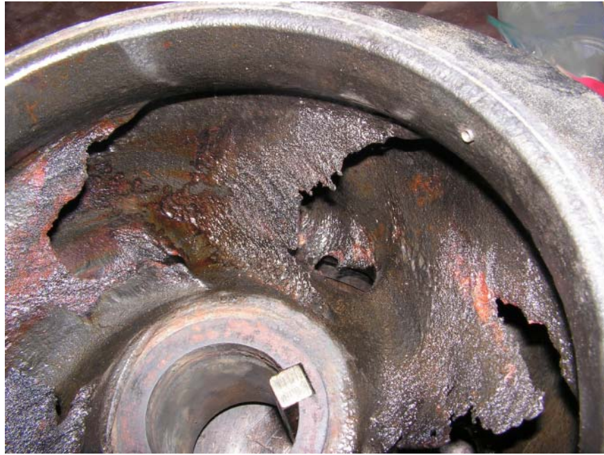
Figure 4-45 – Erosion-Corrosion of is ASTM A48 Class 30 Cast Iron Impeller in recycle water pump.
