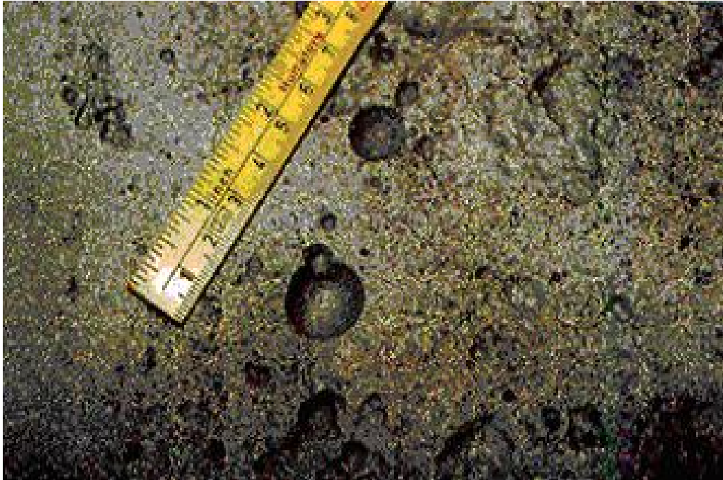
Figure 4-93 – Same oil line as Figure 4-92. Hemispherical pitting typical of MIC can be seen after grit blasting to remove the scale.
