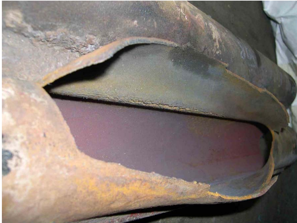
Figure 4-141 – Corrosion fatigue failure of a boiler tube.
