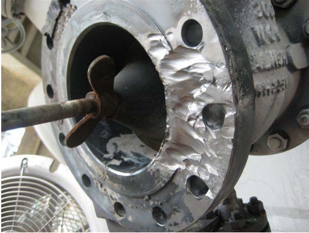
Figure 4-43 – Erosion Corrosion of a 1.25Cr 300 # valve flange on an FCC Catalyst withdrawal line.
