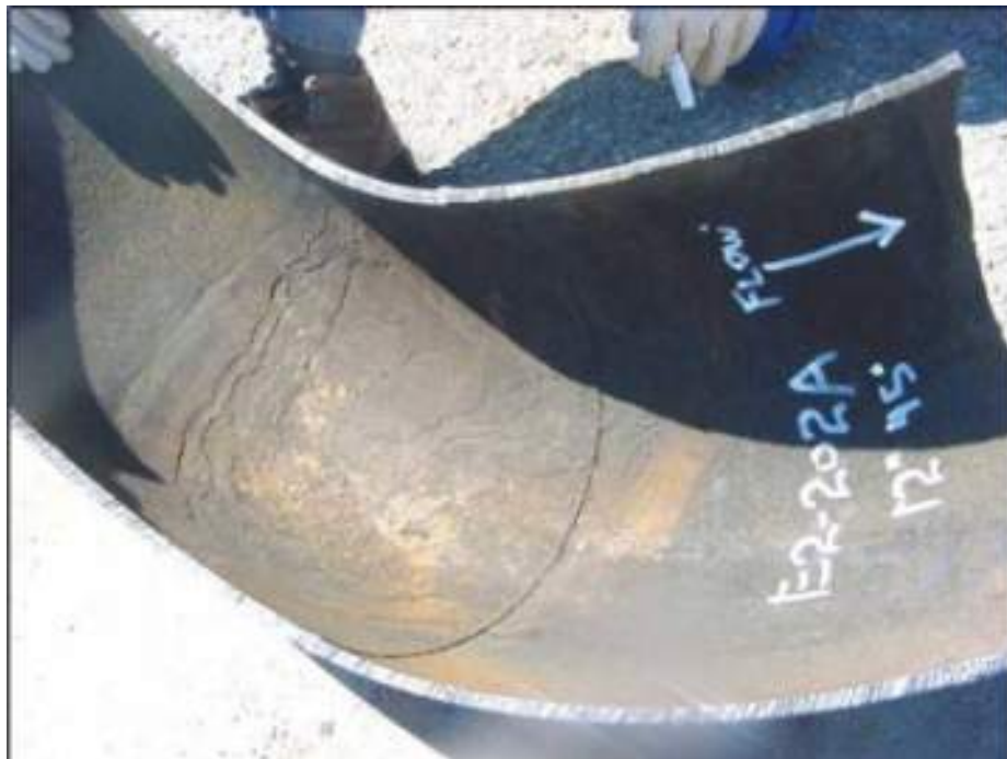
Figure 5-4 – Preferential corrosion in amine regenerator reboiler return elbow (Reference 6).
