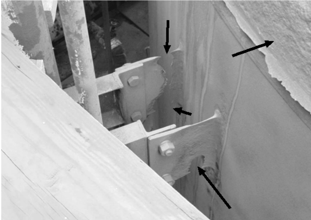
Figure 4-79 – CUI at attachment supports and vessel head.
