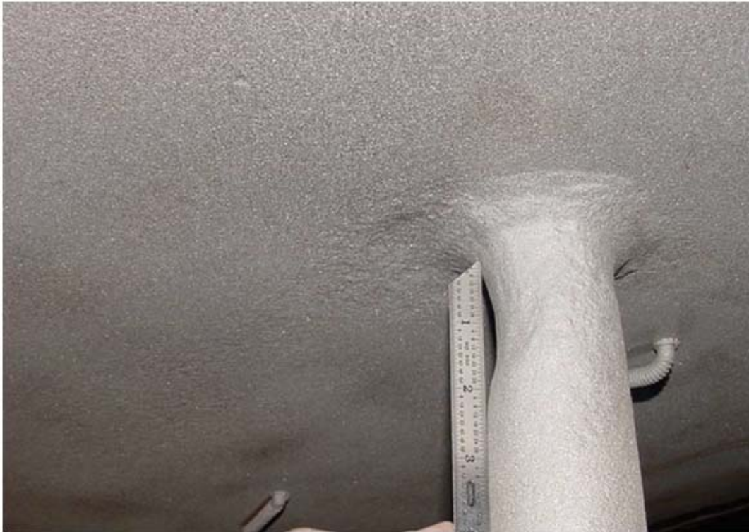
Figure 4-76 – CUI of nozzle on a bottom head.
