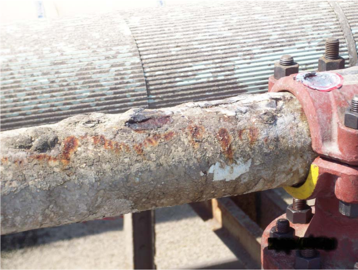
Figure 4-72 – Atmospheric Corrosion of an LPG line in close proximity to a cooling tower.
