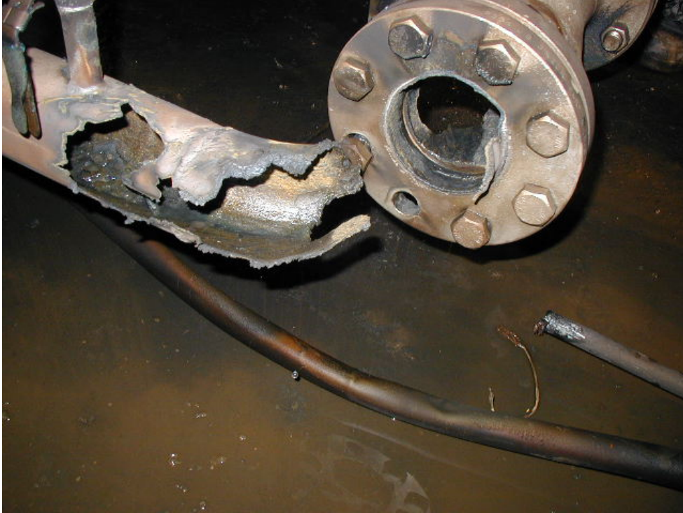
Figure 4-67 – Photograph of a burned 304 SS elbow. The fire started in an upstream stainless steel wire filter (due to particle impact) and the burning filter material impacted the elbow and ignited it. Thin stainless steel components (e.g., filter) are much more flammable than thicker SS. Thin SS (<1/8") is usually avoided in oxygen systems.
