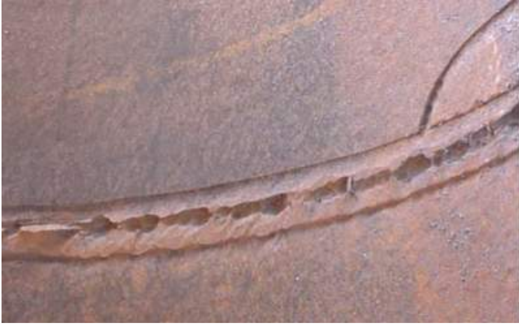
Figure 5-3 – Preferential weld corrosion in lean amine (Reference 5)
