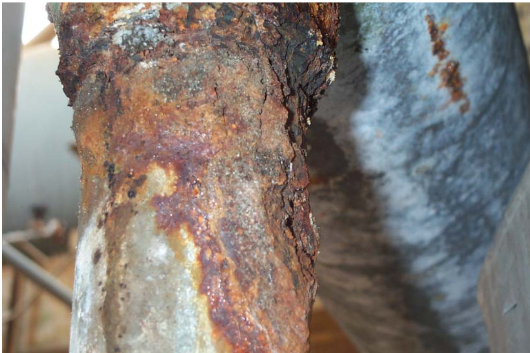
Figure 4-74 – Close-up of Tee CUI of a Tee in Figure 4-73 after insulation removal.
