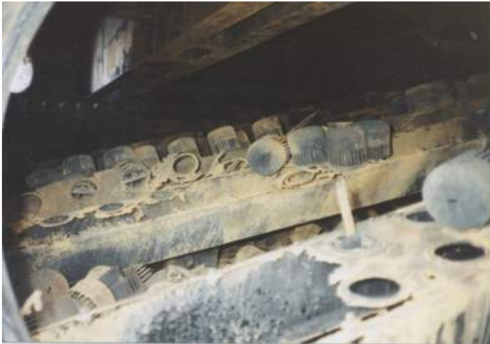
Figure 5-20 – Severe NAC of 410 SS trays and bubble caps in the HVGO section of the vacuum tower fed by the vacuum heater in Figure 5-19.
