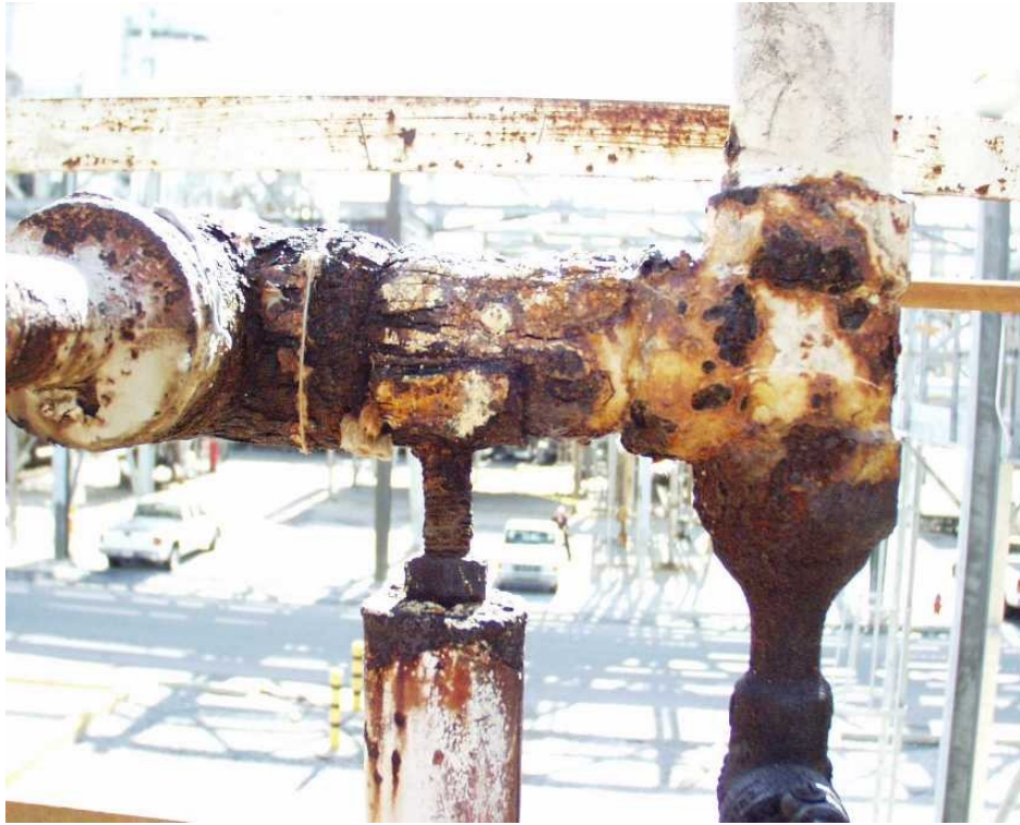
Figure 4-80 – CUI of CS level bridge.
