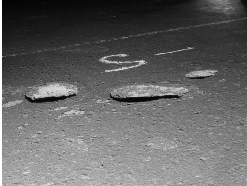
Figure 4-89 – MIC of diesel tank bottom.
