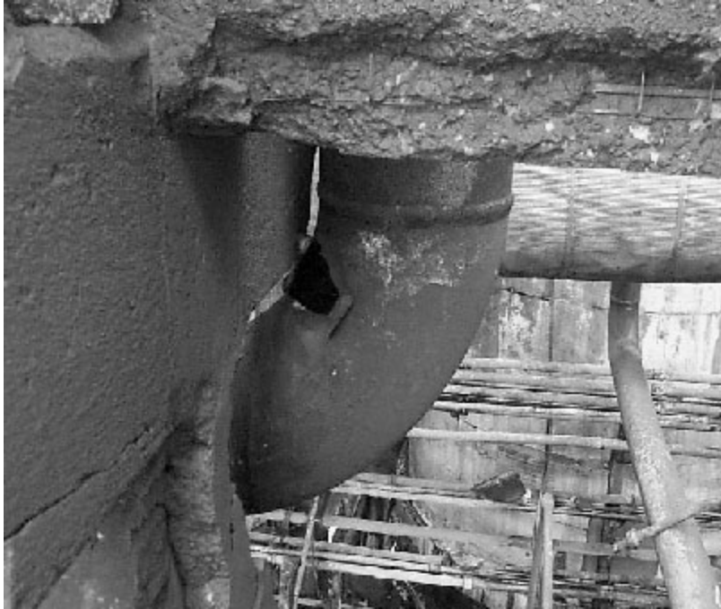
Figure 4-120 – Sulfidation failure of piping elbow.
