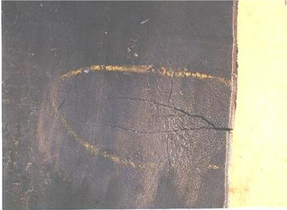
Figure 4-159 – Liquid metal embrittlement of Monel caused by mercury in an FCC gas plant overhead drum.
