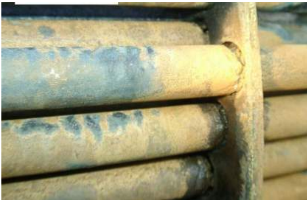
Figure 5-22 – Accelerated corrosion under a baffle.
