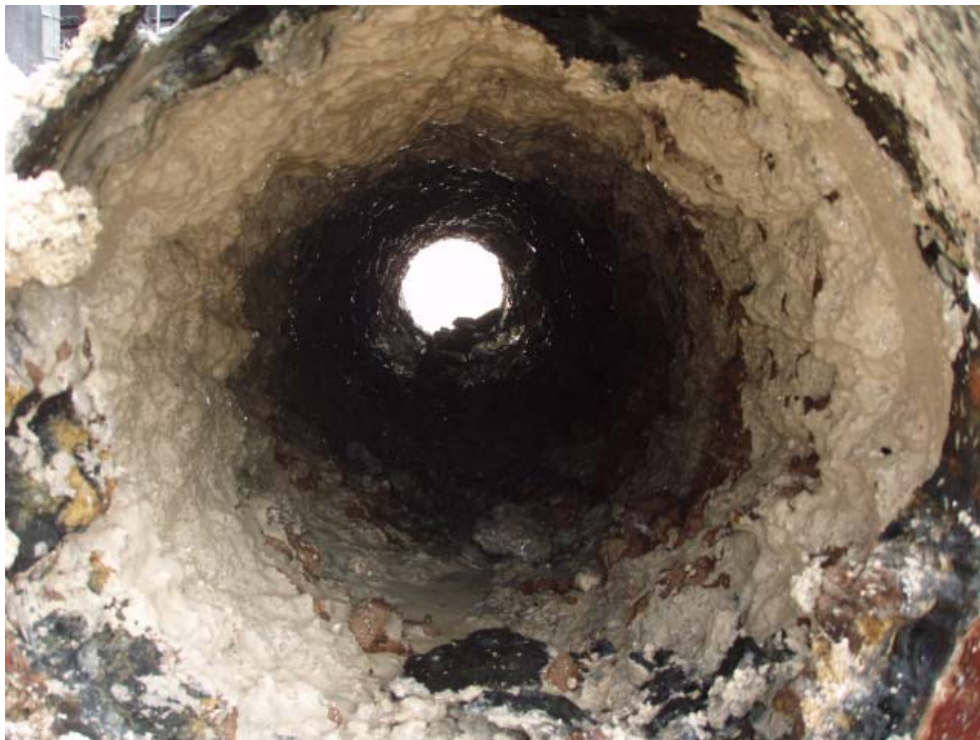
Figure 4-106 – View of concrete lining inside the failed line shown in Figure 105.
