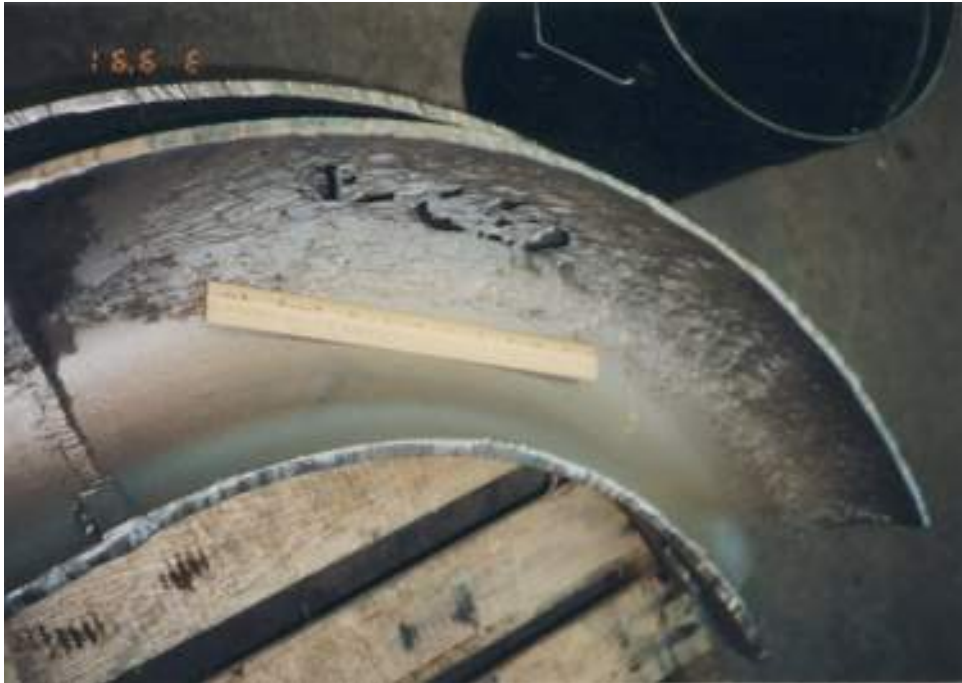
Figure 5-19 – Erosion-corrosion damage due to NAC in a 10-inch 5Cr elbow in the outlet of a vacuum heater in a VDU.
