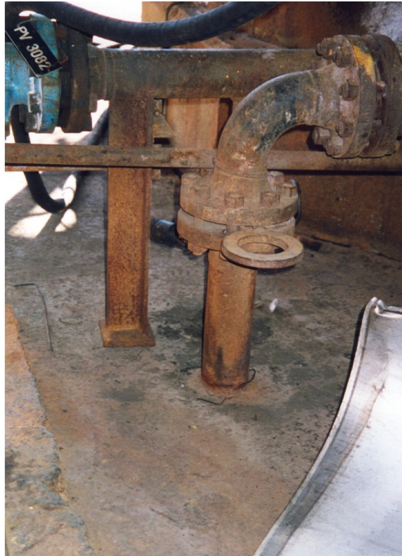
Figure 4-96 – Corrosion of carbon steel pipe at the soil-air interface where the pipe emerges from underground.
