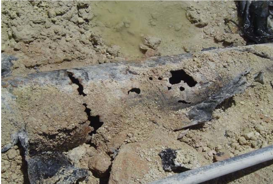
Figure 4-105 – View of the outside of an underground concrete-lined salt water service line that failed from graphitic corrosion.
